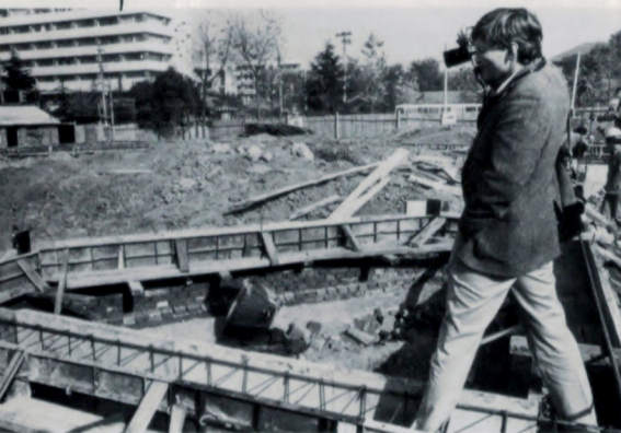
McCracken stands in what will be the projection room in the center's auditorium.
